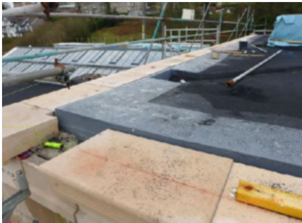
Looking SW: General View – Copings at the SE corner of the Fly tower.
