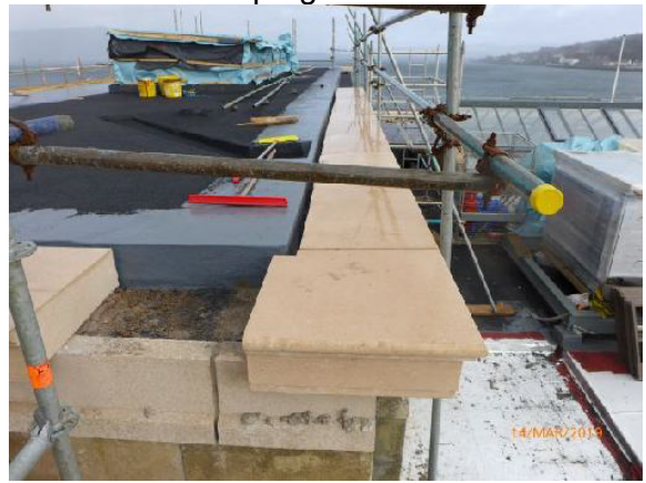
Looking East: General View – Copings at the SW corner of Fly tower.
