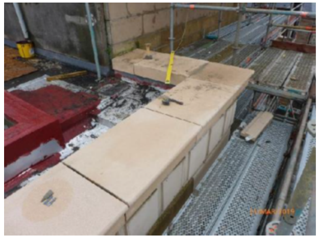
Looking North: General View Installation of the final sections of coping to the Main roof at the NE corner in progress.
