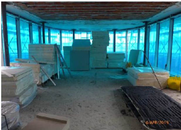
General View of the Exhibition / Function area (the insulation materials stored on the floor are for the Canopy roof above).
