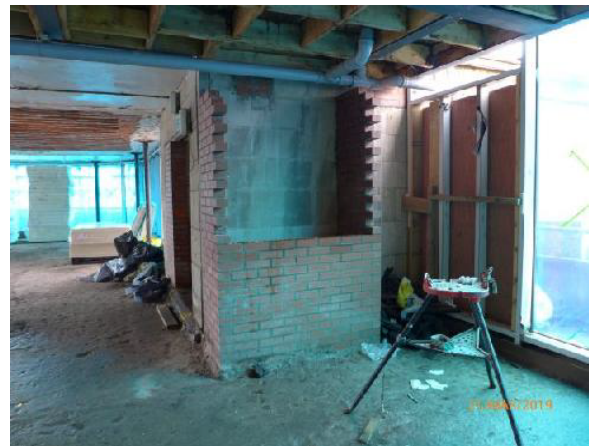
New Office adjacent Staircase (South Elevation – looking East): Brickwork to new service riser.
