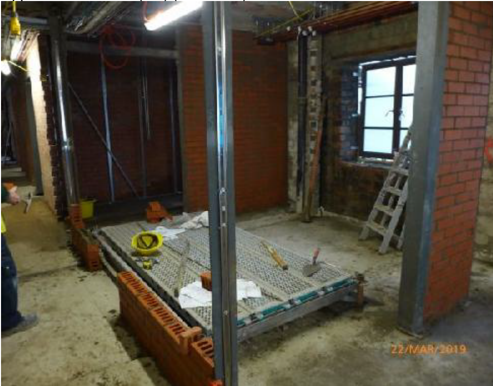
Upper GF – Back of stage area at New Plant room.
