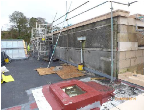
Looking NW: Further Copings now installed to the South elevation of the Fly tower
